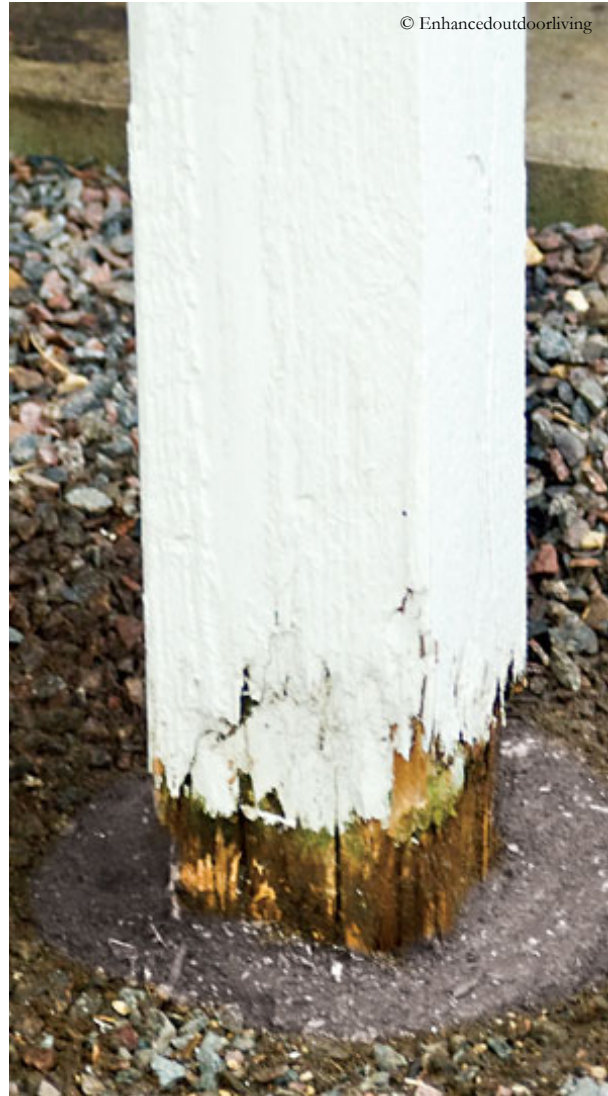
WASSERSCHADEN WATER DAMAGE (Fowing water)
