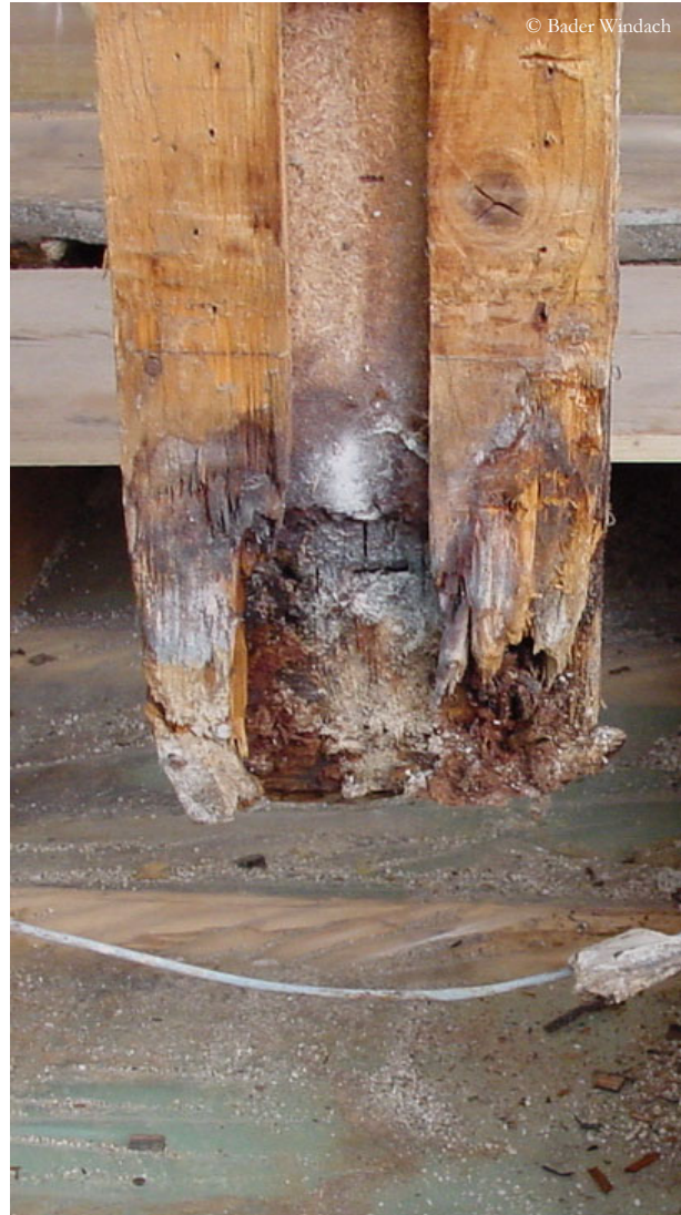
WASSERSCHADEN WATER DAMAGE (High relative moisture)
