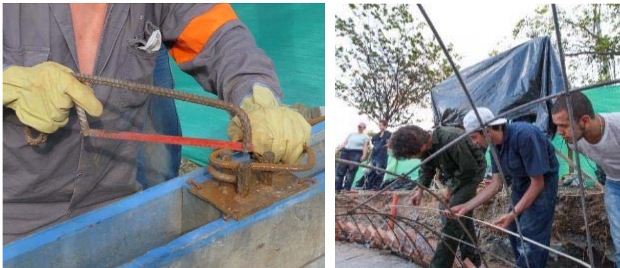
Figure 3: a) One of the worker's improvised handmade tools, and b) student volunteers assisting with the construction (© Sergio González).
