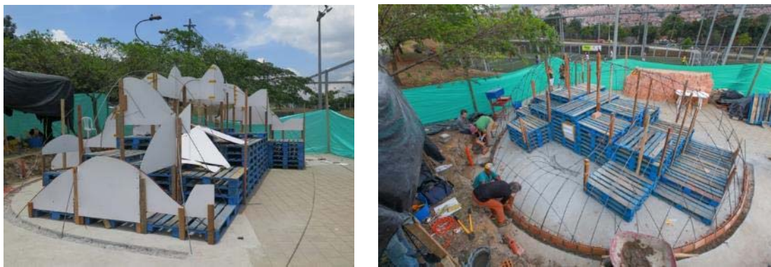
Figure 7: a) Construction of the falsework with cardboard sections and the studs as guides, rebars were bent in place; and b) the finished falsework (© Sergio González).
