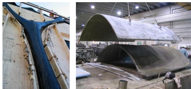
Figure 2: (left) Fabric formwork for a beam with expressive, natural curvature [4]. (right) Simple vault cast on fabric formwork [4].
